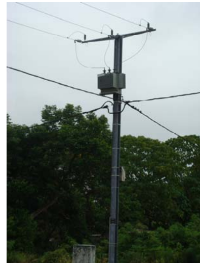
Transformer, Luganville (Source: IPA)
