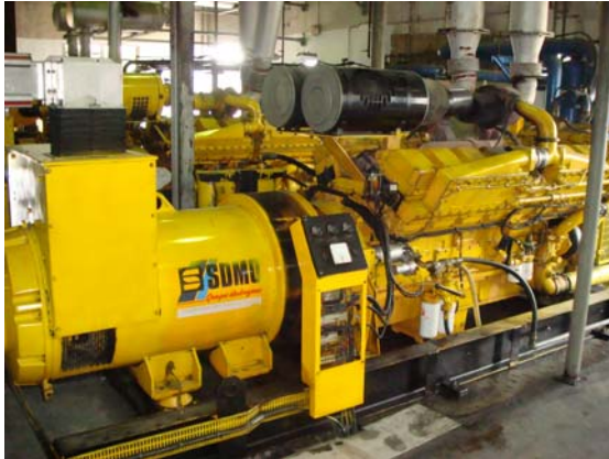
Diesel generating unit, Luganville (Source: IPA)
